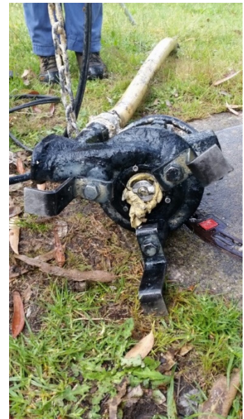
A blocked sewer pump
