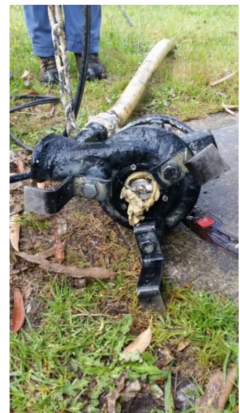
A blocked sewer pump
