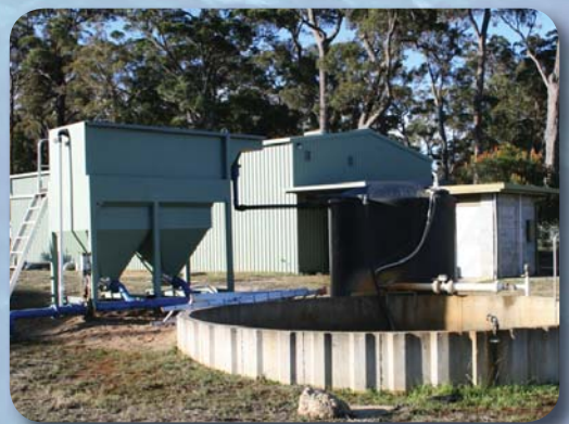
Earmarked for upgrades: Bairnsdale Wastewater Treatment Plant (top) and the water treatment plant at Mallacoota
