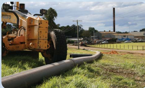
Laying out sections of new sewer main on the outskirts of Bairnsdale before installation underground
