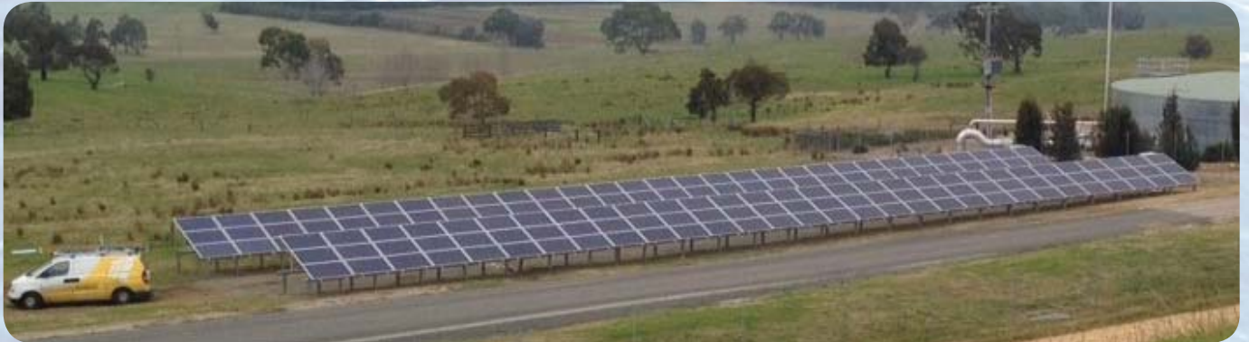
A bank of highly efficient solar panels just installed at Woodglen Water Treatment Plant will greatly reduce the running costs of the facility
