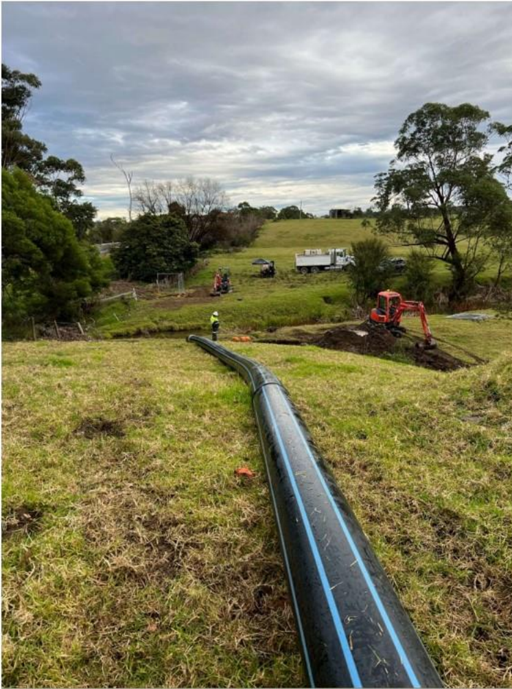
Caption: The new welded HDPE water main 'pipe string' being prepared for installation under Youngs Creek, Orbost.
