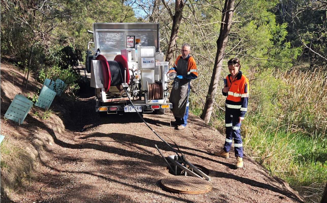
Image shows the sewer blockage being jetted as part of East Gippsland Water's emergency response.
