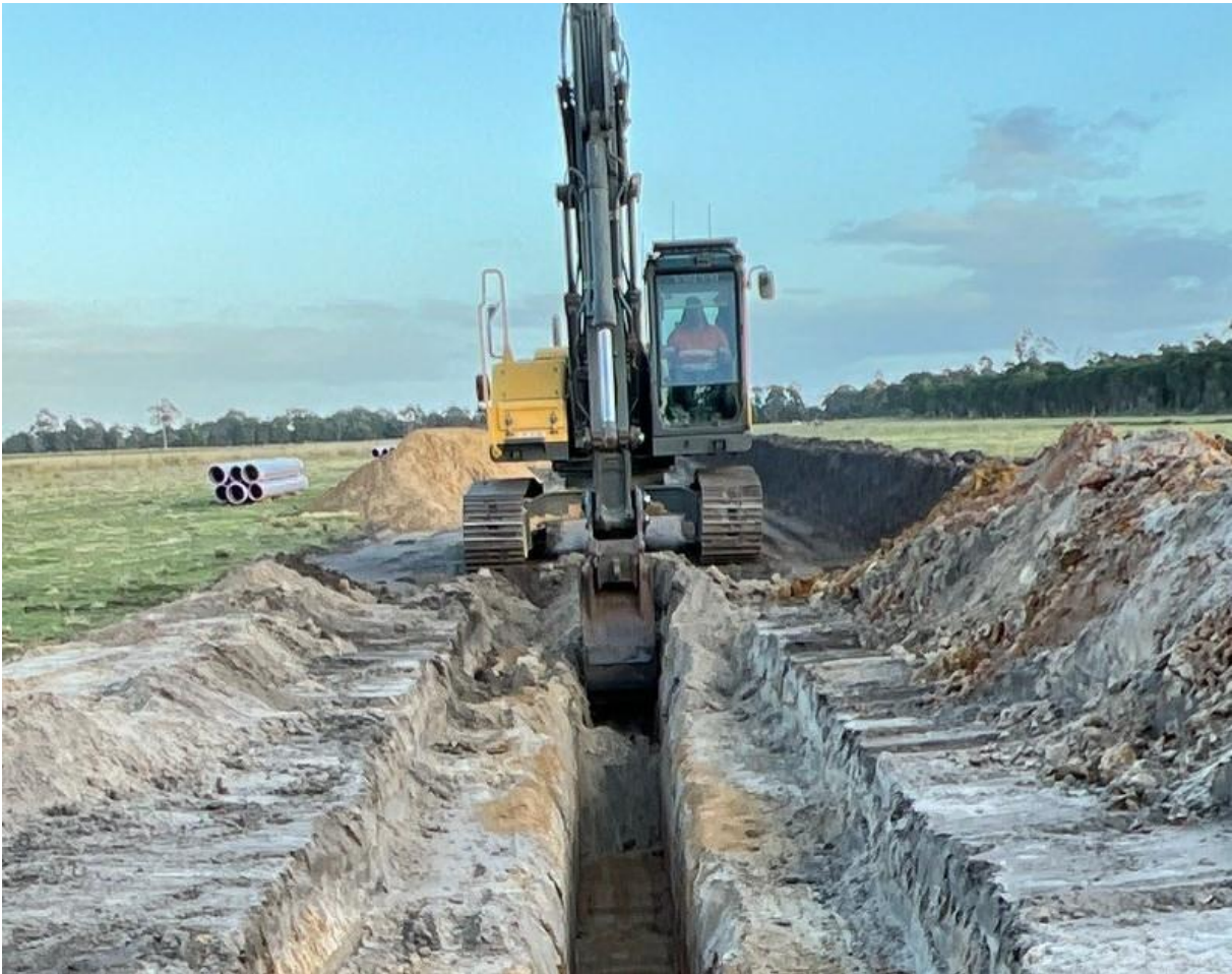
Image shows work commencing on the first section of the 3,000 metre Ring Main Trench
