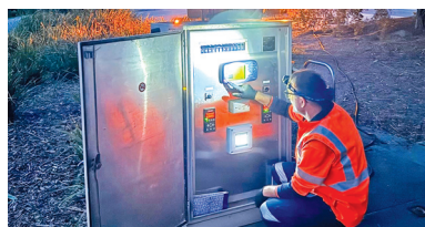
One of our controls and systems team members, Dino, at the Metung Sewer Pump Station
