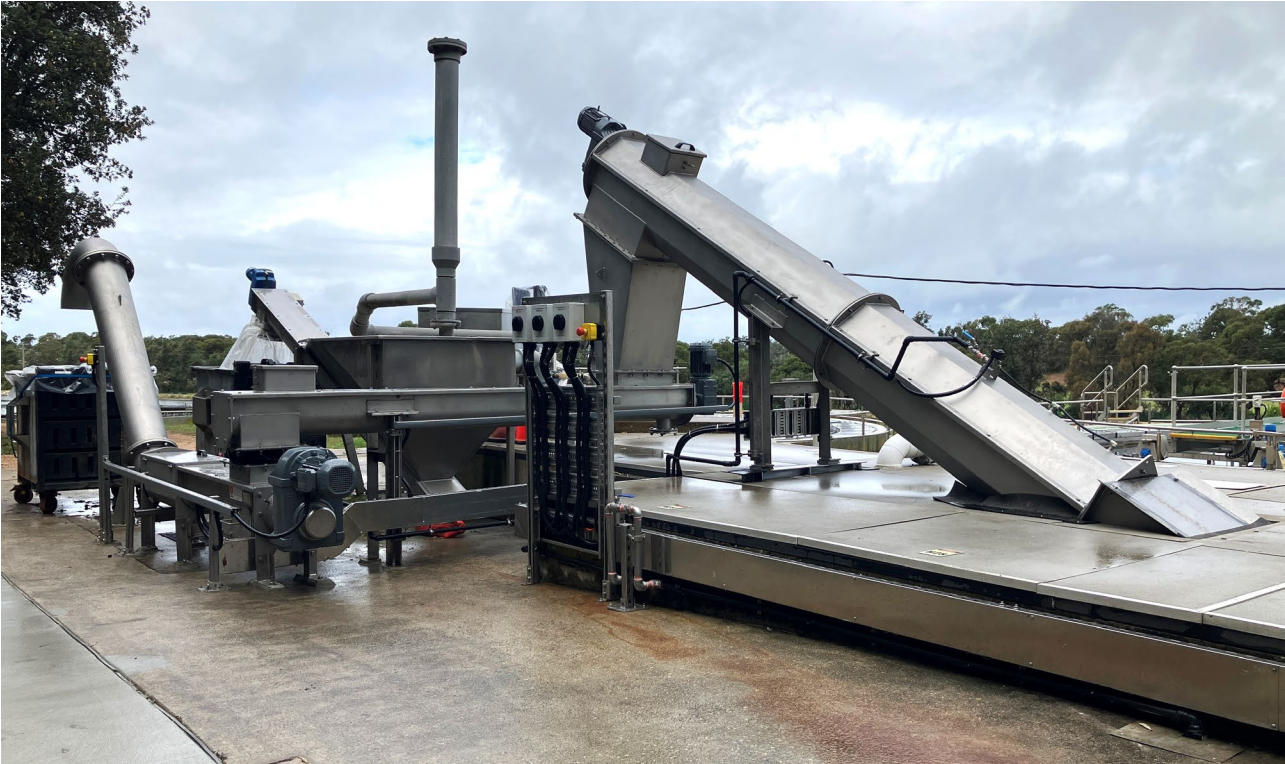
The image shows the new inlet screen, transfer conveyor and wash press at the Lakes Entrance Water Recycling Plant
